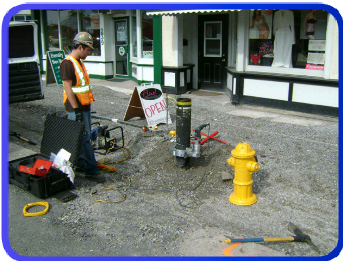
Remove hydrant and install the Wachs' portable split frame cutting and grooving machine
