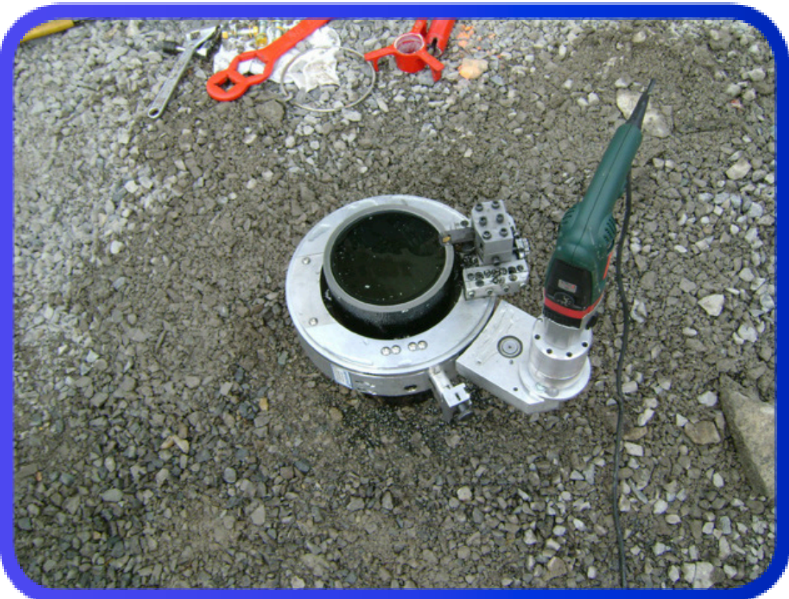
The hydrant pipe is cut and prepped to mount at the correct grade
