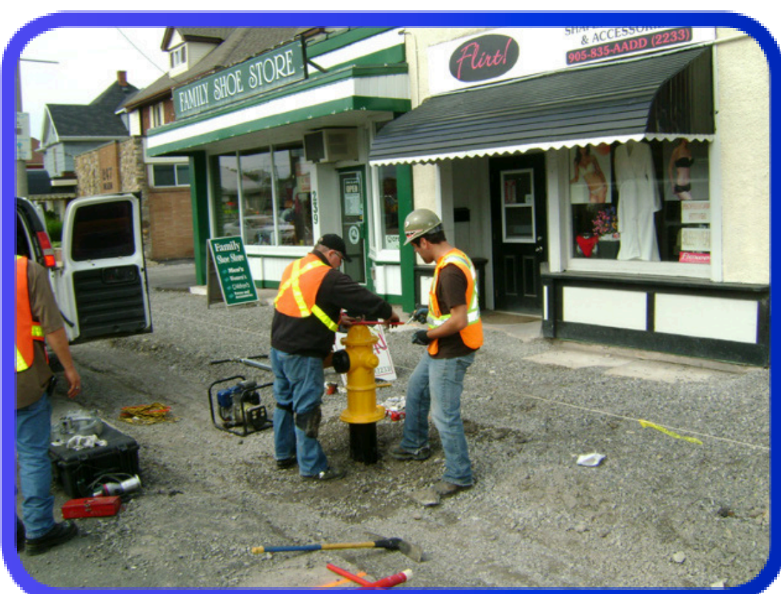
Remove Wachs machine and reinstall the original hydrant at it's new grade level
